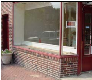
Vacant storefronts detract from the streetscape presence in the historic downtown core
