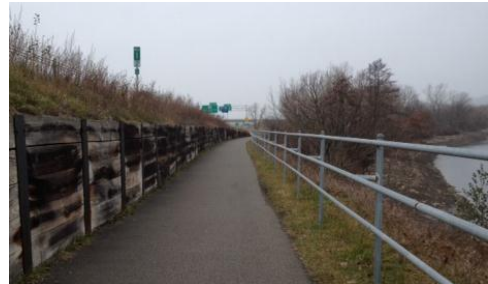
Example of a shared use path cut into the side of a roadway embankment along I-890 in Schenectady, NY.
