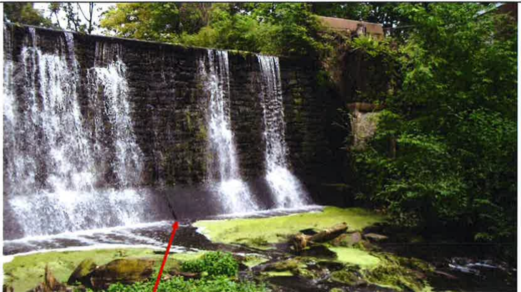
Misalignment of splash apron
